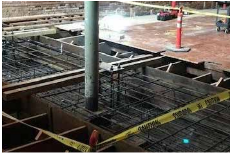
Foundation work: The foundation is being reinforced to ensure the structural integrity of the historic building.
